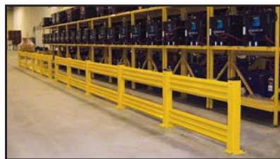
Guarding Battery Racks
