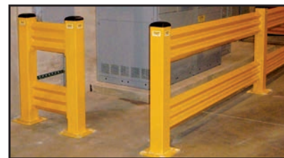
Guarding Electrical Panels
